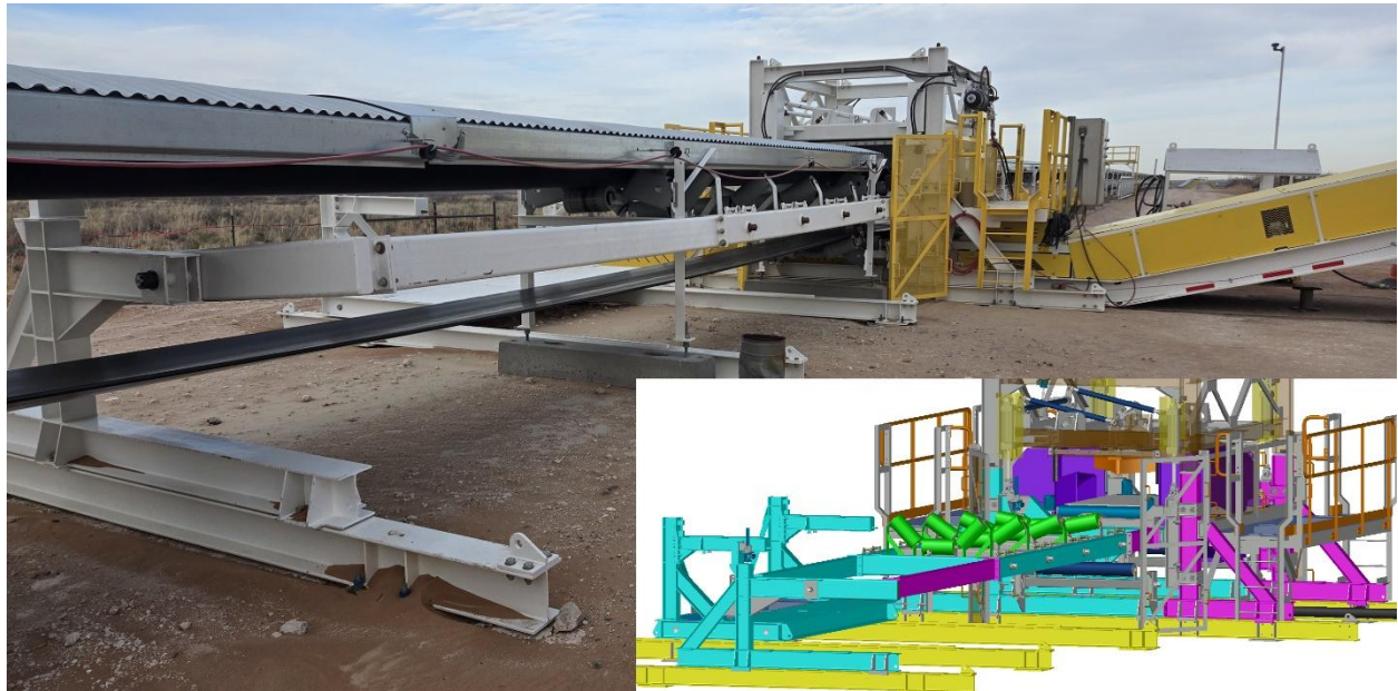
Figure 10: Mobile Plow Station installation enveloping standard ground modules with a low-profile belt feeder (inset showing 3D model of the plow station mechanism)
