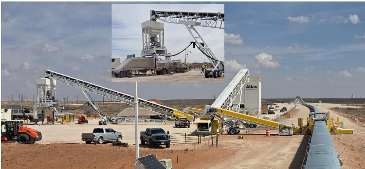
Figure 9: Mobile off-load plow station installed on a horizontal curve along 120-CV-004
