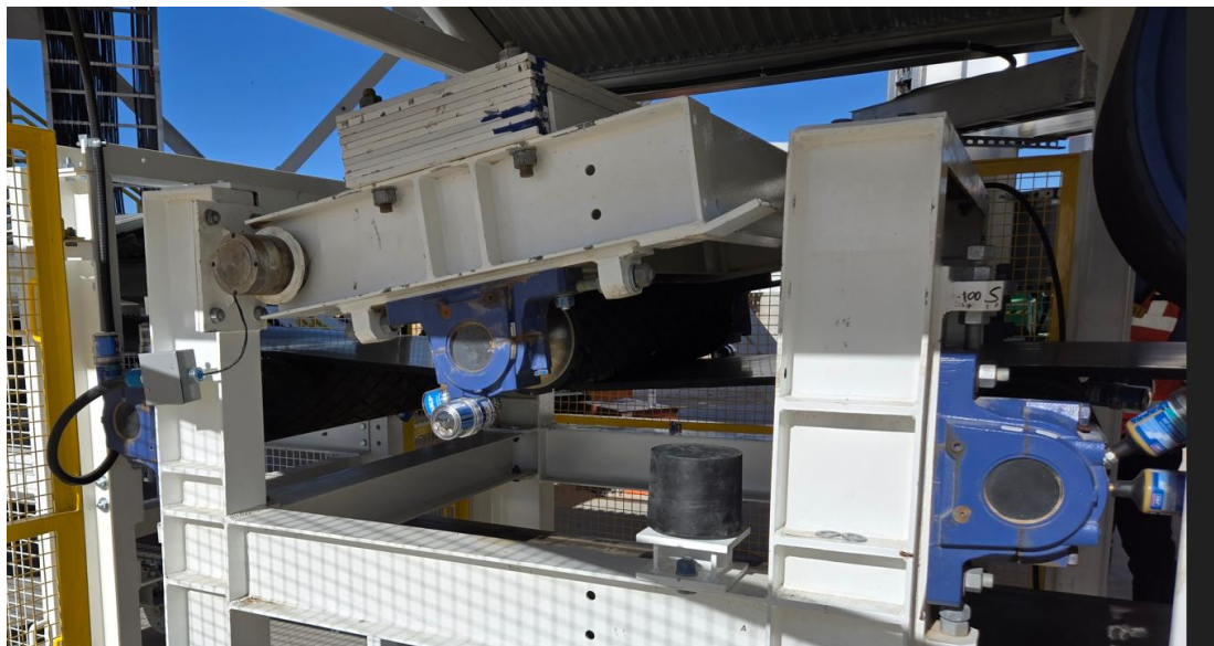
Figure 4: Rotary Encoder based Belt Tension Measurement for Tail Drive Control
