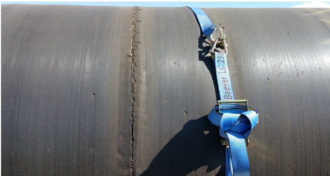
Figure 2. Roll of belt removed with a split in excess of 100m
