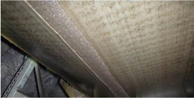
Figure 1. Bottom Cover Idler Junction Failure in Longwall Retraction conveyor
