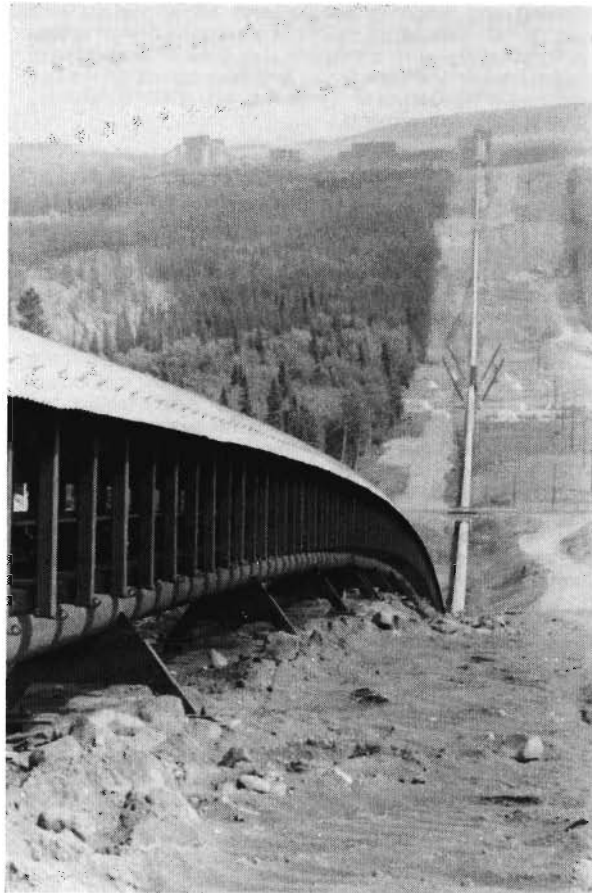
Figure 2 The C2 downhill conveyor at the Quintette Coal mine in British Columbia, Canada, is 7 km long and uses a single DC drive and hydraulic disk brakes.
